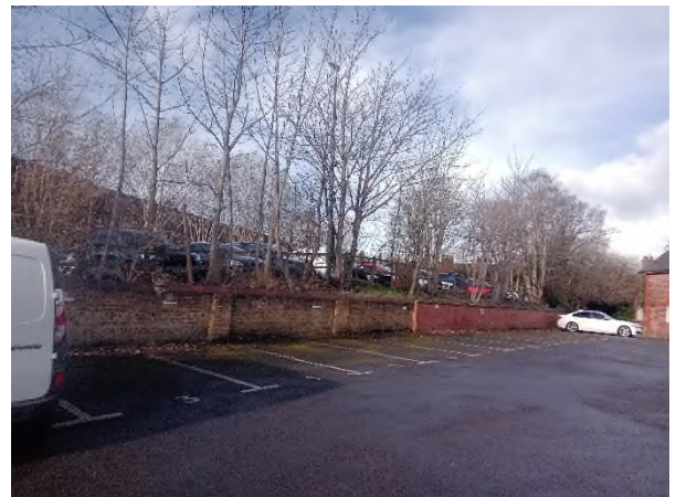
Figure 2.6: Retaining wall on eastern site boundary. Photograph taken from the Caledonian Car Park.
